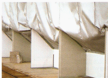
The custom-made fire curtain spanned 160m (top); curtain sections were bolted to floor angles and then stapled together (above)
