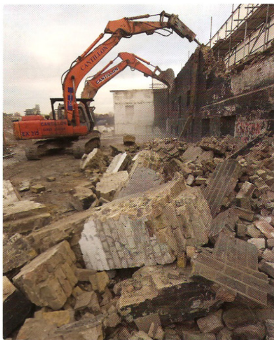
Figures 3 (right) and 4 (below): The walls of the building are carefully pulled down under close supervision and brick, stone and concrete is amassed on-site before being taken away for recycling.
